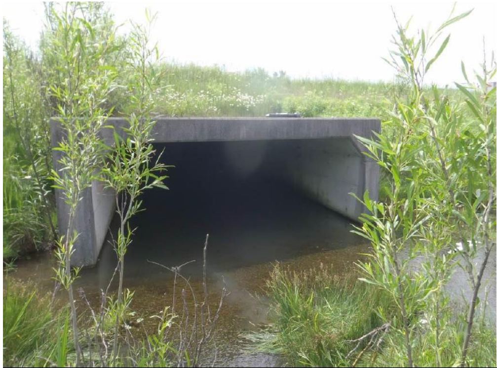
Photo 1 – Tributary to Murray Drain (Site No. 19-650c): At Murray Drain culvert upstream of culvert; facing downstream (south)
