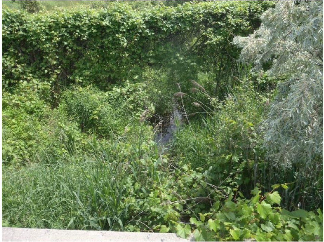
Photo 7 – Elliot Laidlaw Drain (Site No. 19- 351/c): At upstream side of culvert facing downstream (south). Note vegetation
