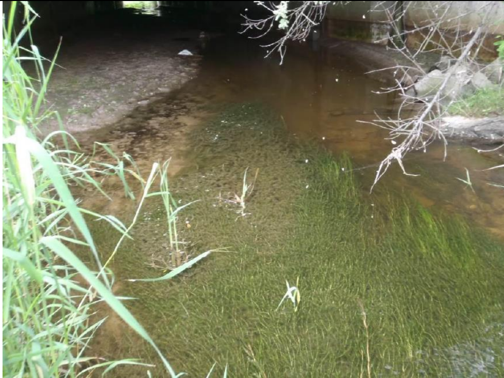
Photo 4 – Elliot Laidlaw Drain (Site No. 19- 351/c): At upstream side of culvert facing downstream (south). Note vegetation
